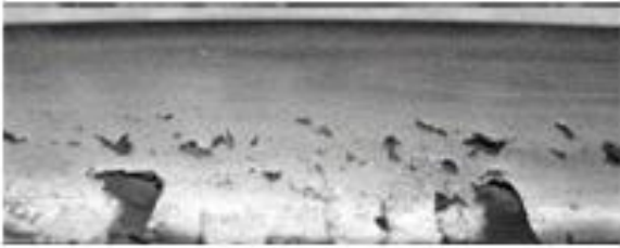
Figure 2. Railway track with spalling
