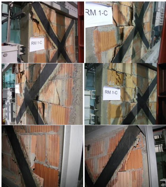
Fig. 6 Failure mode for RM1-C (RM1-strengthened)
